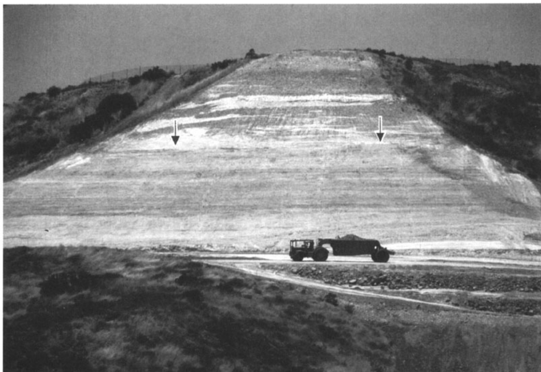
Figure 4. View of Highway 52 cut slope looking north. BPS (arrows) occurs in a thin claystone bed within a sequence of Eocene sandstone and conglomerate.
